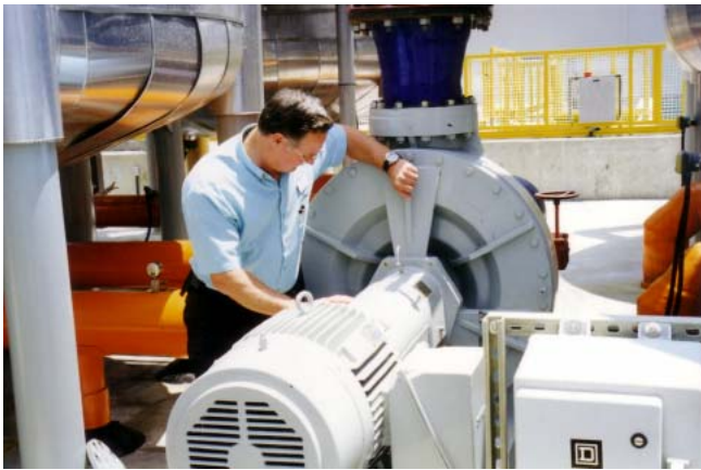
Fybroc carbon filter pump. It pumps 6,000 gallons per minute of salt water. It is protected with LE's 6413 LOW TOX Turbine Oil.
