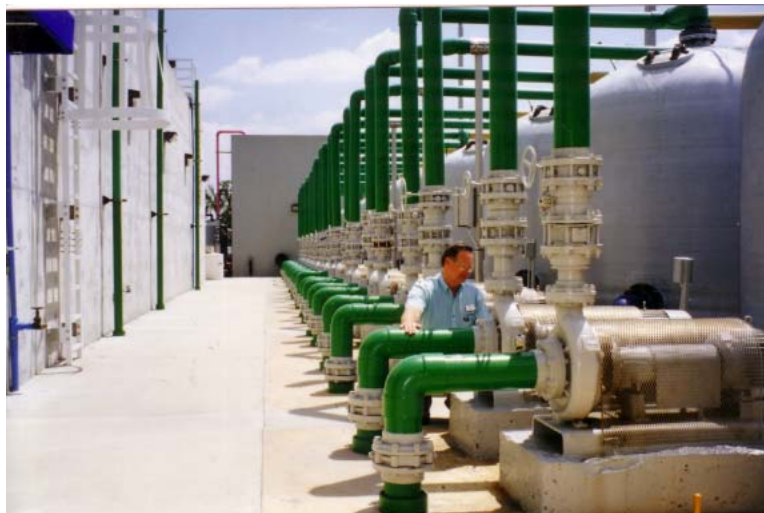
20 main plant filtration pumps 700 GPM each of salt water
